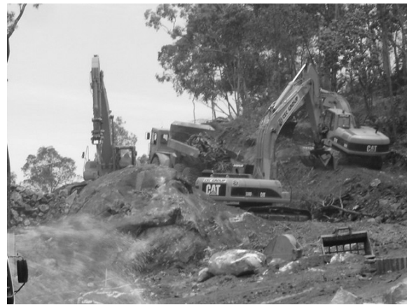
Some of the current destruction - photo by Nev Ridley
