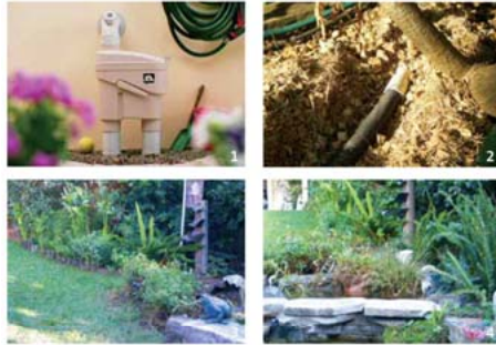
Greywater is diverted from a shower using a licensed diversion device (1) and distributed directly to citrus and water-loving plants through a slotted pipe (2) under 100mm of mulch. In this unusual installation, a small portion of the flow is diverted through a series of six gravel filterbeds (3) which remove nutrients and pollutants. After five days in the filterbeds, the water enters two water-feature fish ponds (4) with gravel filters to further polish the water.
